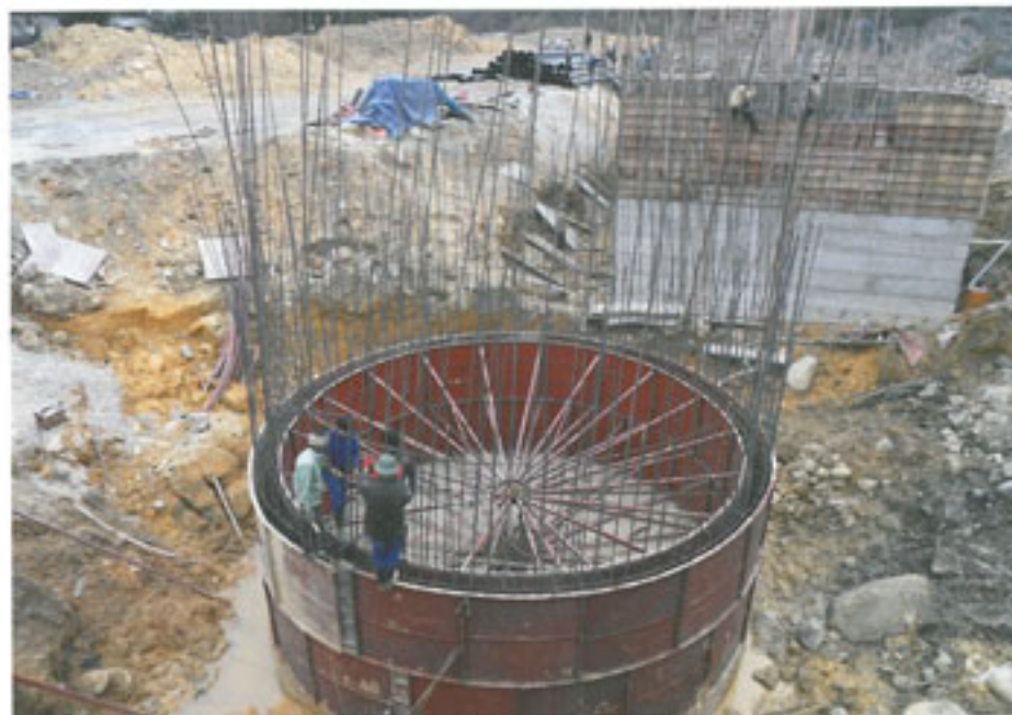
PLANT CONSTRUCTION: Sludge thickener (front) and sedimentation basin (back) of the first expansion stage (January 2011)
